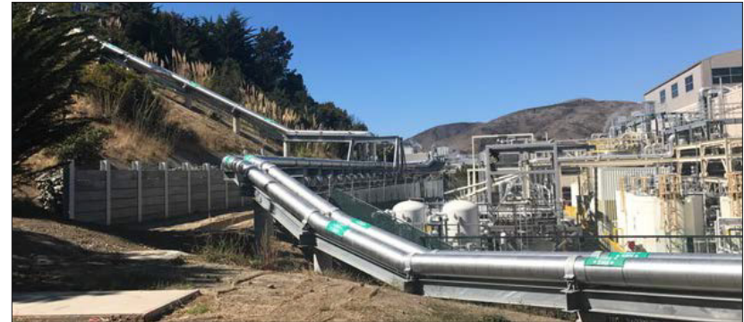
Genentech On-Site Systems
